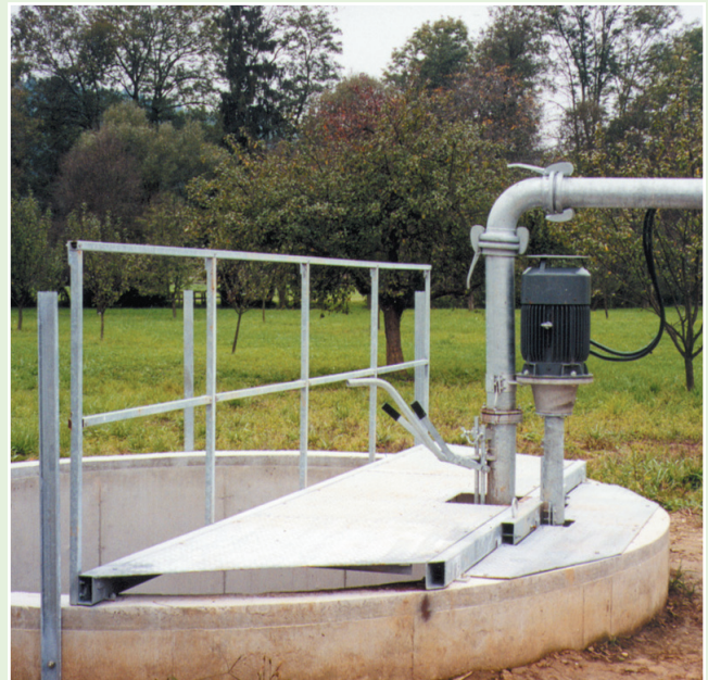
Permanently installed LE model used for transfer
