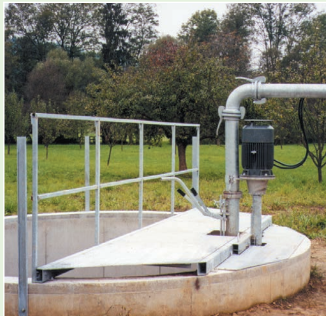
Permanently installed LE model used for transfer
